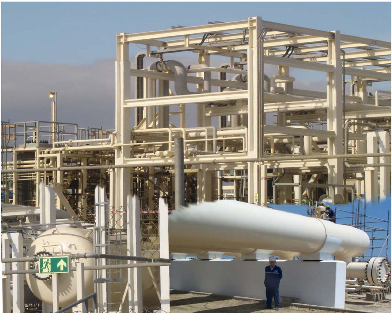
Figure 1. Right; Sales Manager Geoff Robinson stands beside concrete plinth in the Slug Catcher Area and left and above; steel structure. All protected with Cafco's Fendolite MII system.
